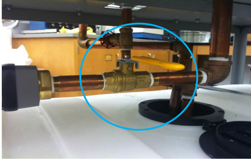
FIGURE 49. Valve installed to control rate water flow into liquefaction tank.
