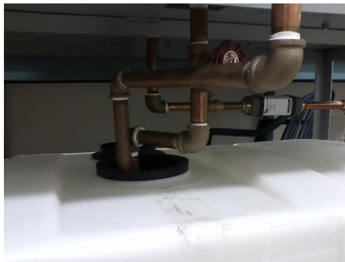
FIGURE 54. Overflow drain directed into water reservoir.
