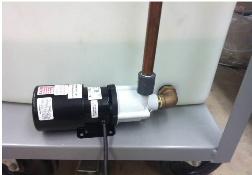
FIGURE 47. Water pump connected to the tank and outlet pipe installed with plastic coupling.
