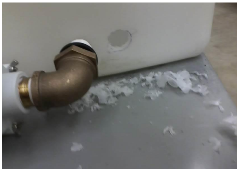
FIGURE 45. Hole drilled on side of reservoir tank for installation of pump inlet.
