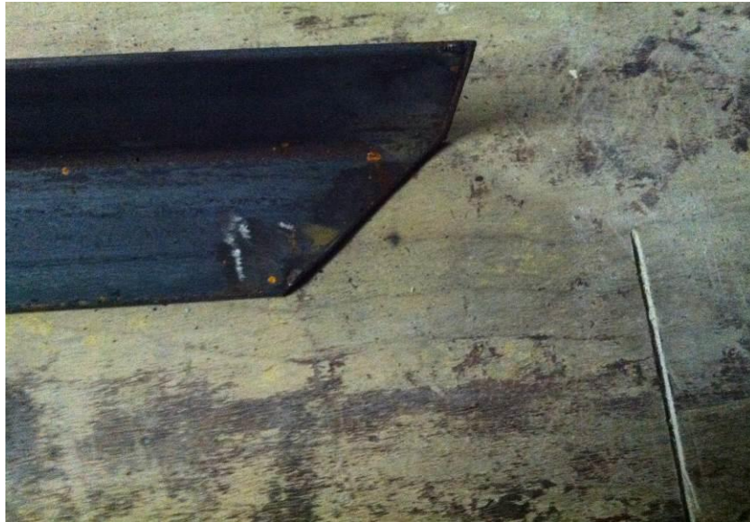
FIGURE 24. Angle steel ends cut to 45 degrees to allow for welding of a square base.
