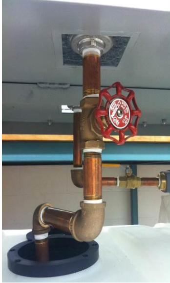
FIGURE 51. Tank drainage pipe system with control valve.
